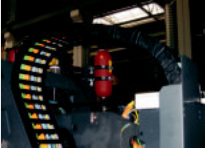
Series E4.42 in a machine tool, completely assembled with igus® Chainflex® cables
