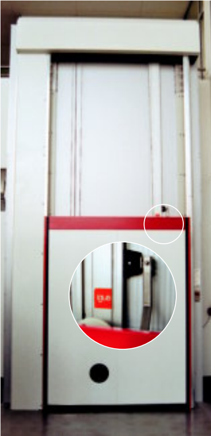
Energy supply to the strip at cold storage house doors, in operation for more than one year.
