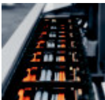
Orderly laid cables with igus® interior separation
