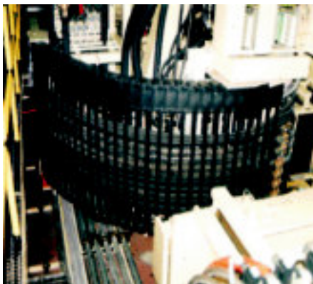
Hydraulics and electric cables are separated from one another in this example
